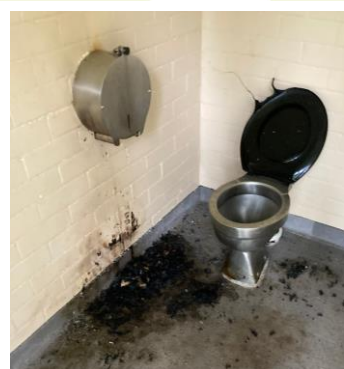
Public Toilet infrastructure burnt
