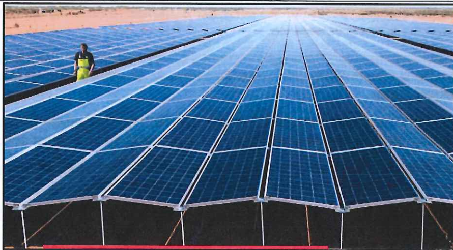
Figure 3.1.b Source Belectric – Installed example of PG PV Plant system
